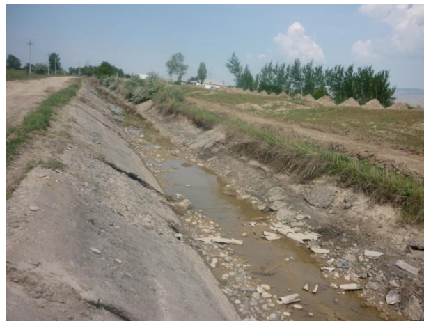
Bad Bad irrigation canal before rehabilitation
