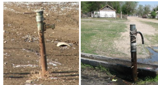
Remains of old potable water systems at Keneral (left) and Maulenbay (right) villages
