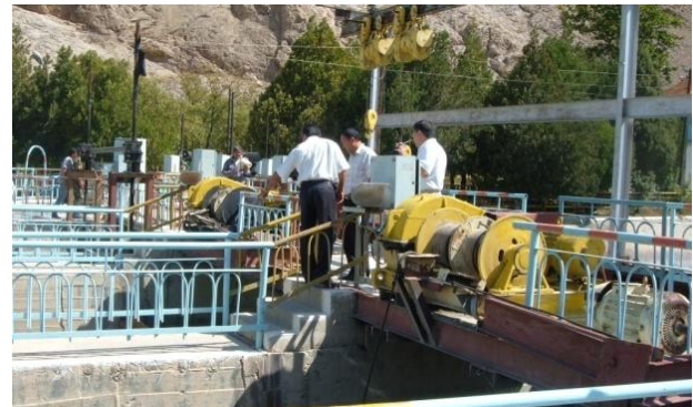
A radial gate hoist at the headwork’s main body
