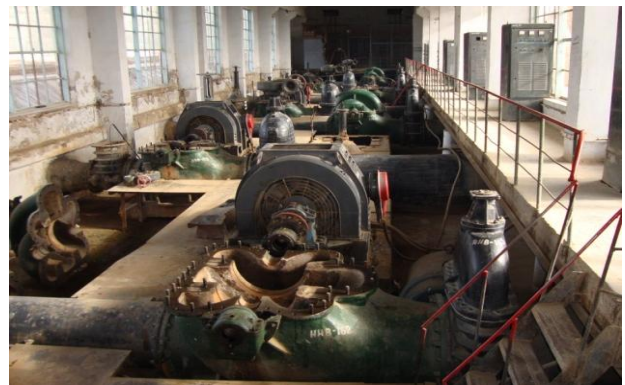
A cascade of five pump stations supplied irrigation water to lands around Garauti
